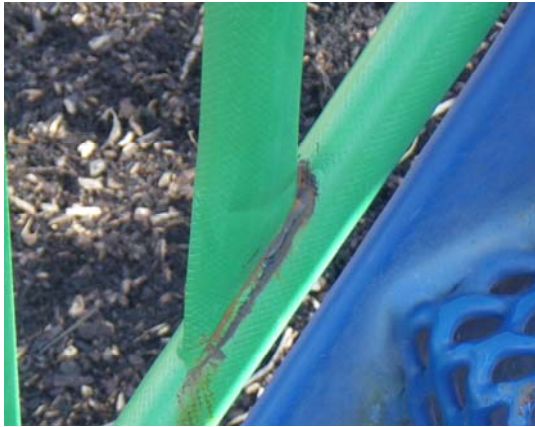
Failing Weld on railing
