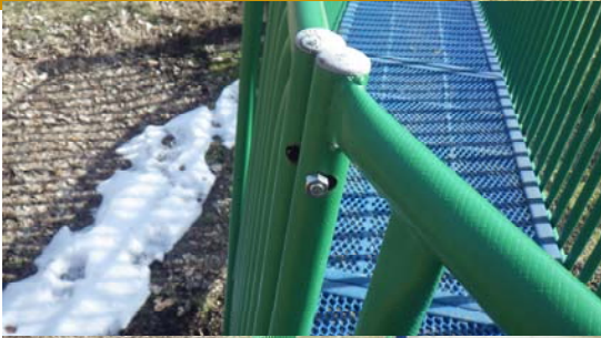
Repairs done due to replacement parts not being available
