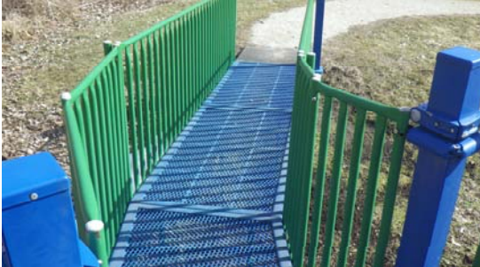
Non-ADA compliant ramps
